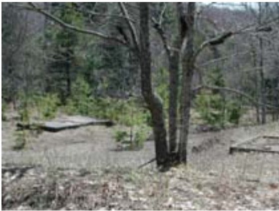
The cracked stone foundations at Camp AuTrain are typical of those found at all of the camps today. In many cases, the concrete foundations are hidden under the leaves and branches of trees, bushes and other vegetation, which has overgrown the former POW camps. This photograph was taken in autumn 2002. (Photograph by John Pepin)
